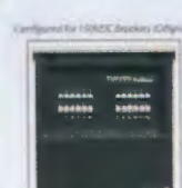
Configured for 150VDC breakers (Offgrid)
