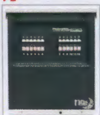
Configured for 150VDC breakers (Offgrid)
